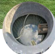
Lamellar settler solid separation.
