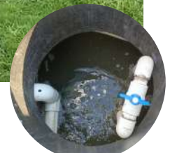
Disinfection system. Reactor to disinfect by ozone.
