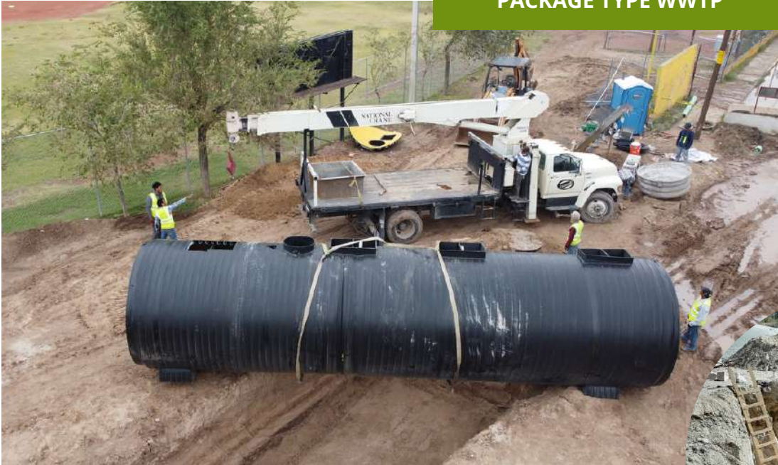
PACKAGE TYPE WWTP
