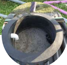
Reactor 1 MBBR. Organic matter removal reactor.
